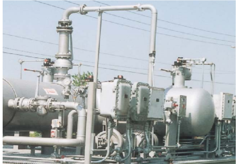
Mixing and Analyser system
